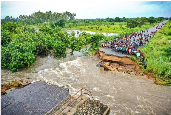
Figure 1. Bridge collapsed isolating communities in central Mozambique due to cyclone Gombe in 2022. Photo: INGD
